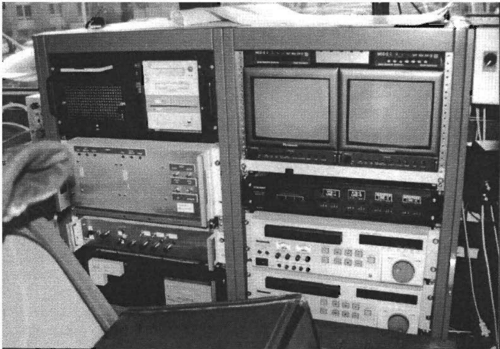
Figure 9. Properly Mounted Electronic Equipment.
