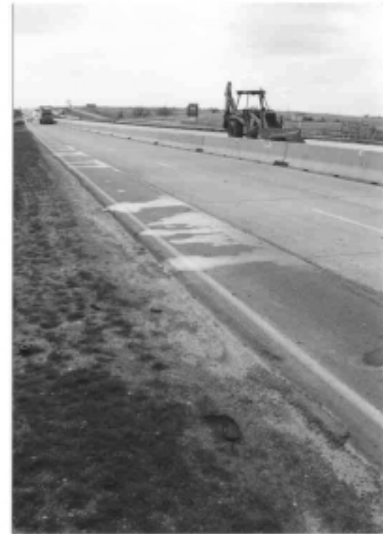
Vertical Moisture Barrier near Palmer, Texas. Barrier installed at edge of asphalt shoulder 8 foot deep. Moisture seeping from concrete/asphalt joint.
