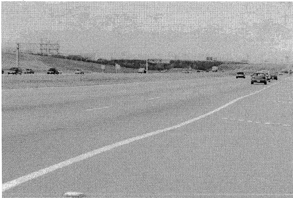
Figure 11. Sections of IH 635 Experiencing Heaving
