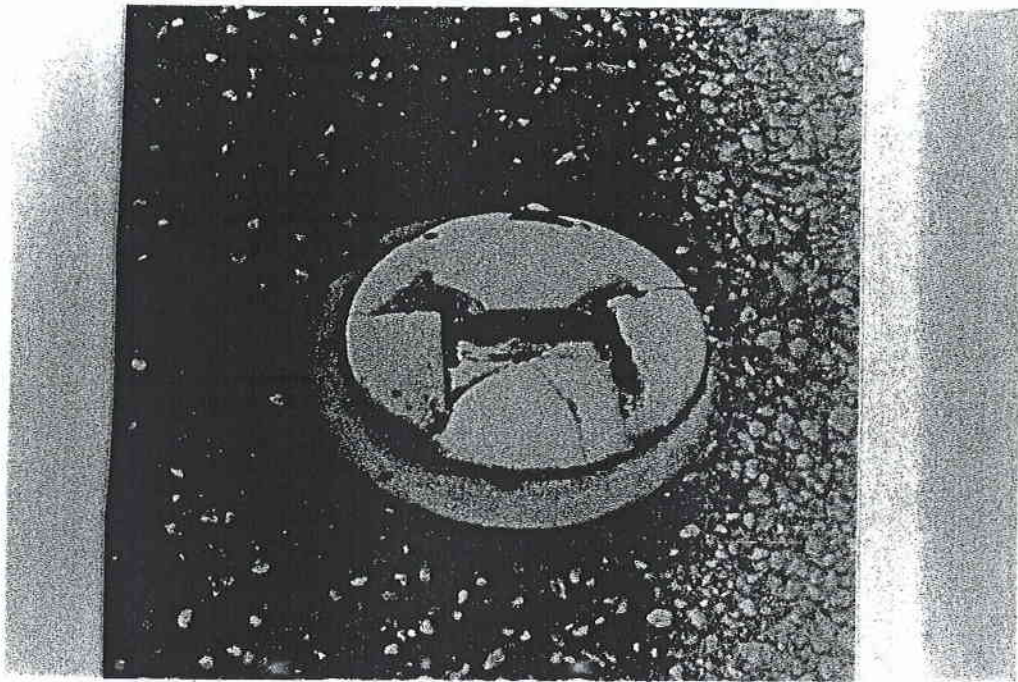
Figure 13. RTB, Type I-C, Badly Broken and Worn. Lens is Completely Missing.
