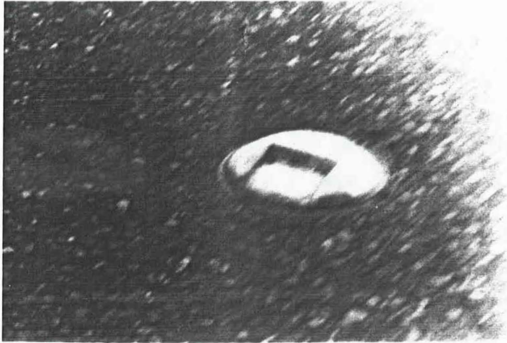
Figure 13. A RTB Submerged Into the Asphalt Pavement.
