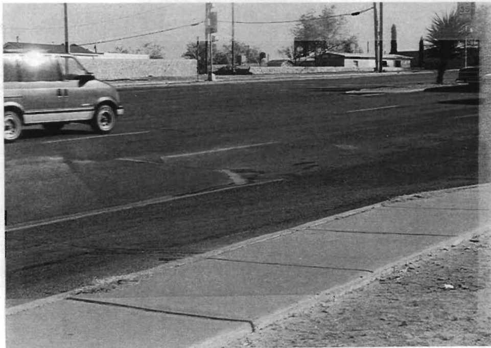
Figure 27. Water Seeping from Pavement Near the Intersection with Kern Street.
