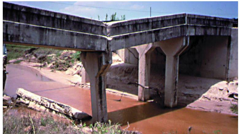
Scour-erosion of the stream bed-causes serious damage to bridges every year
