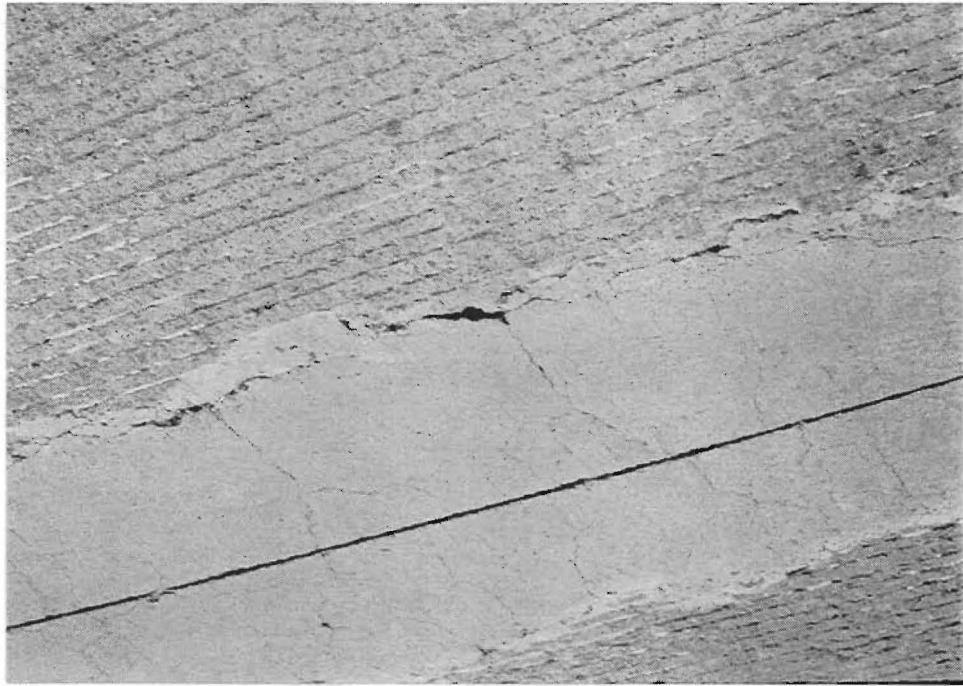
Fig. 3.6. Debonding and Map Cracking Observed on October 20, 1993.
