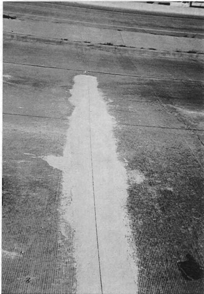
Fig. 4.7. An Extended Spall Repair with a Saw Cut.
