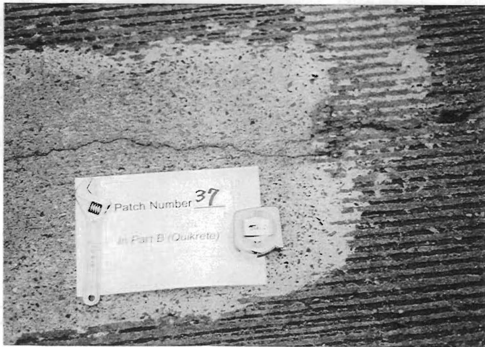
Fig. 4.10. Repair No. 37: A Transverse Crack on the Uncut Patch (January 4, 1995).
