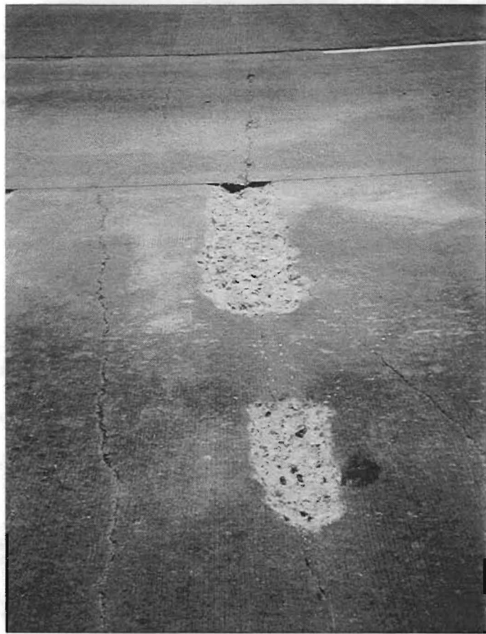
Fig. 4.5. Spalling Spots Before Filling of Repair Mixture.
