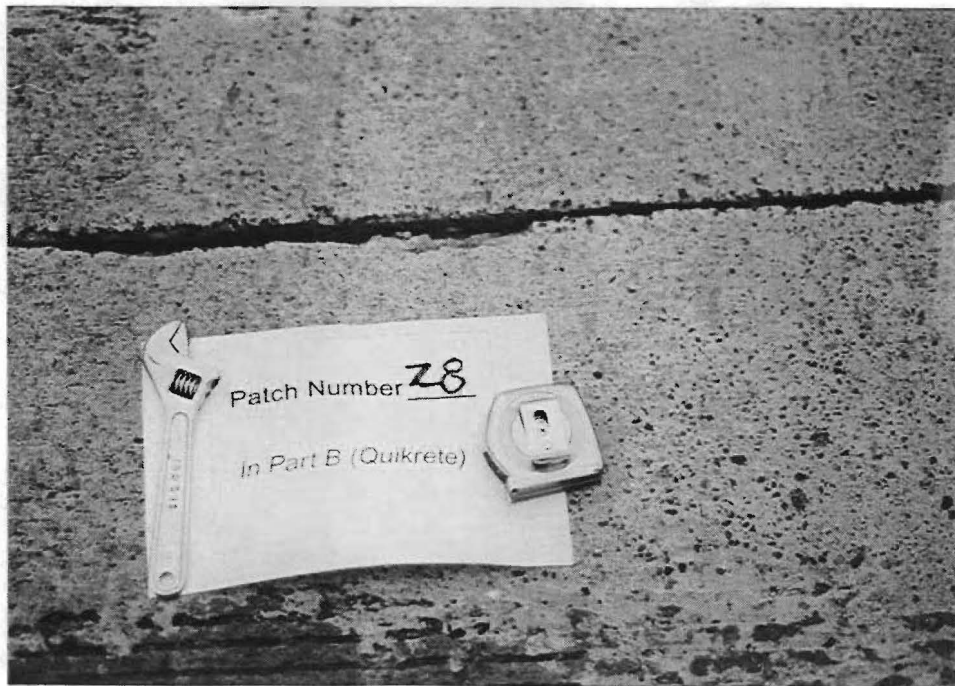
Fig. 4.8. Repair No. 28: Minor Spalling Along The Saw Cut (January 4, 1995).
