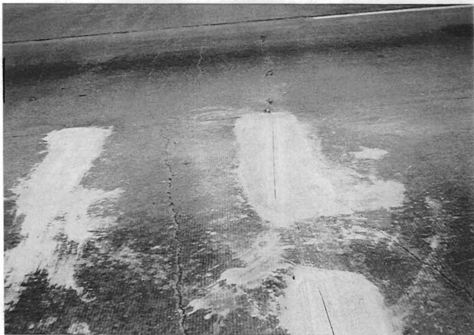
Fig. 4.6. Spalling Spots After Repairing and Saw Cutting.
