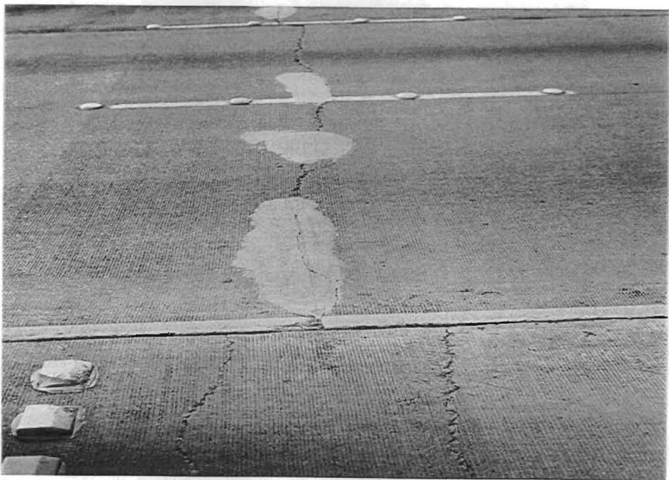
Fig. 3.7. Transverse Cracking and Minor Spalling (January 20, 1995).
