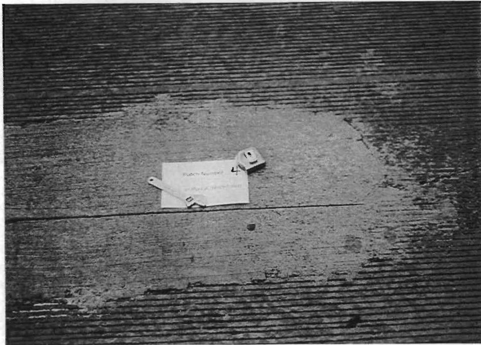
Fig. 4.11. Repair No. 4: No Random Crack on a Saw Cut Patch (January 4, 1995).
