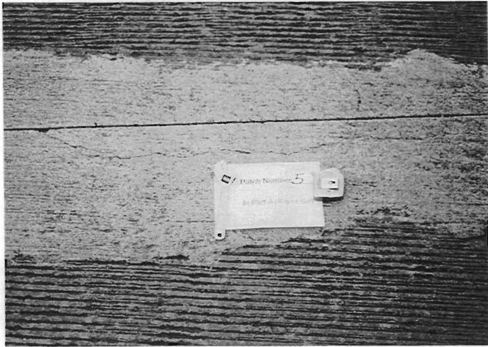
Fig. 4.9. Repair No. 5: A Transverse Crack Near the Saw Cut (January 4, 1995).
