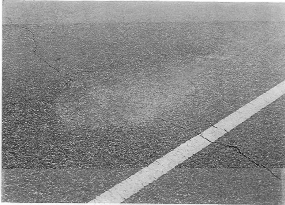
Figure 1. Transverse Depressions in the Wheel Path (Note Pumping of Fine Material).
