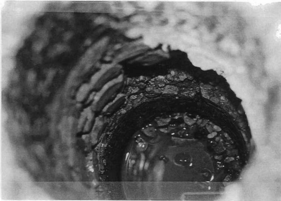
Figure 3. Core Hole with Disintegration of the Top 150 mm of the CTB Layer.
