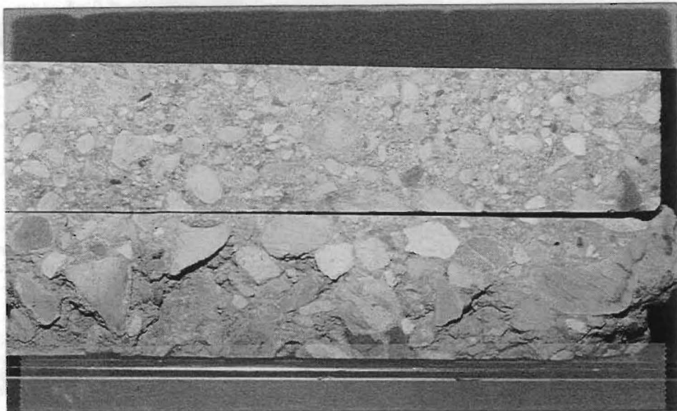
Figure 1.2. In situ Sample from SH 36 Shows the Bottom Half of the Cement Treated Base Deteriorated More Rapidly than the Top Half.
