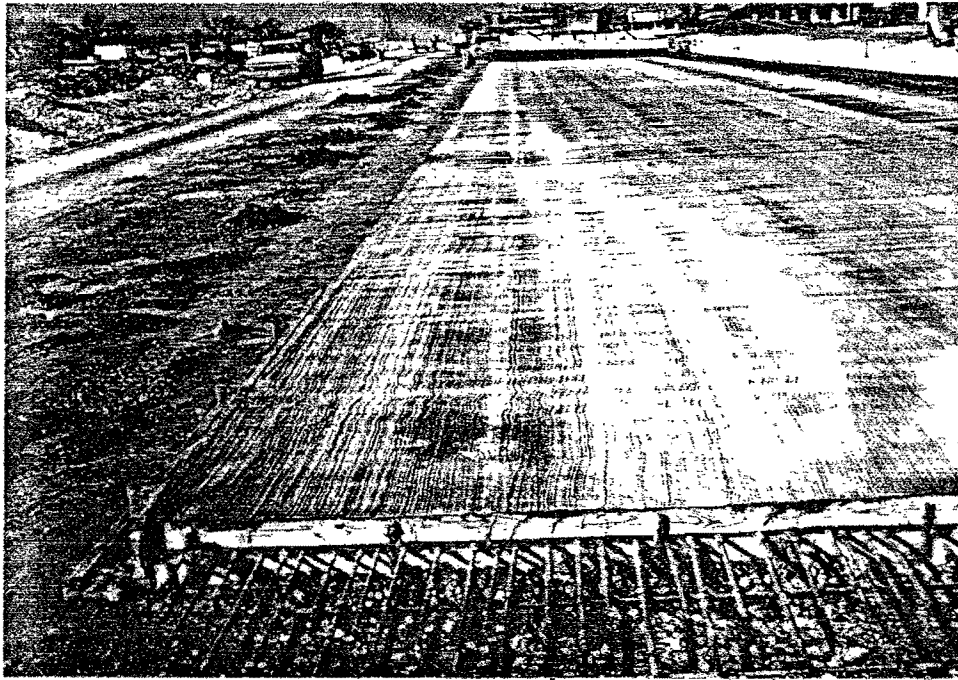
Figure 27. Finished Concrete Pavement showing curing compound on Loop 12, Dallas Co. (Test Site 11).
