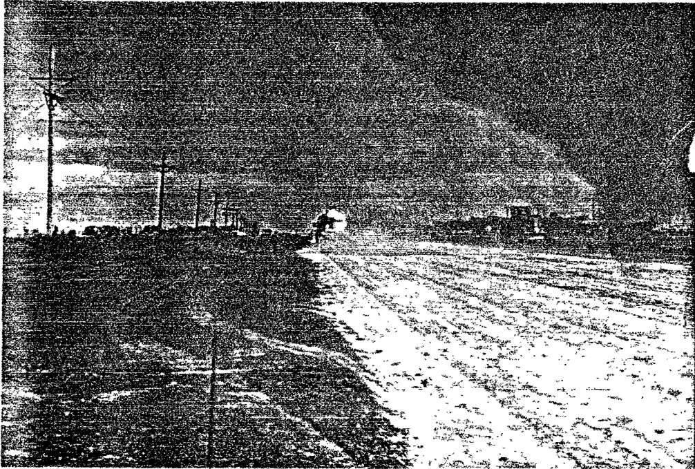
Figure 13. Application of Fly Ash on SH 335 in Amarillo, Texas (Test Site no. 8)
