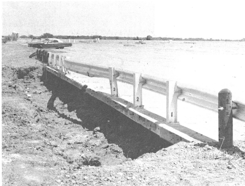
Figure 14. TUBULAR W-BEAM Bridge Rail after Crash Test 1B. (Note 0.61 m (2.0 ft) residual lateral deflection. Posts 4, 5 and 6 broke away.)
