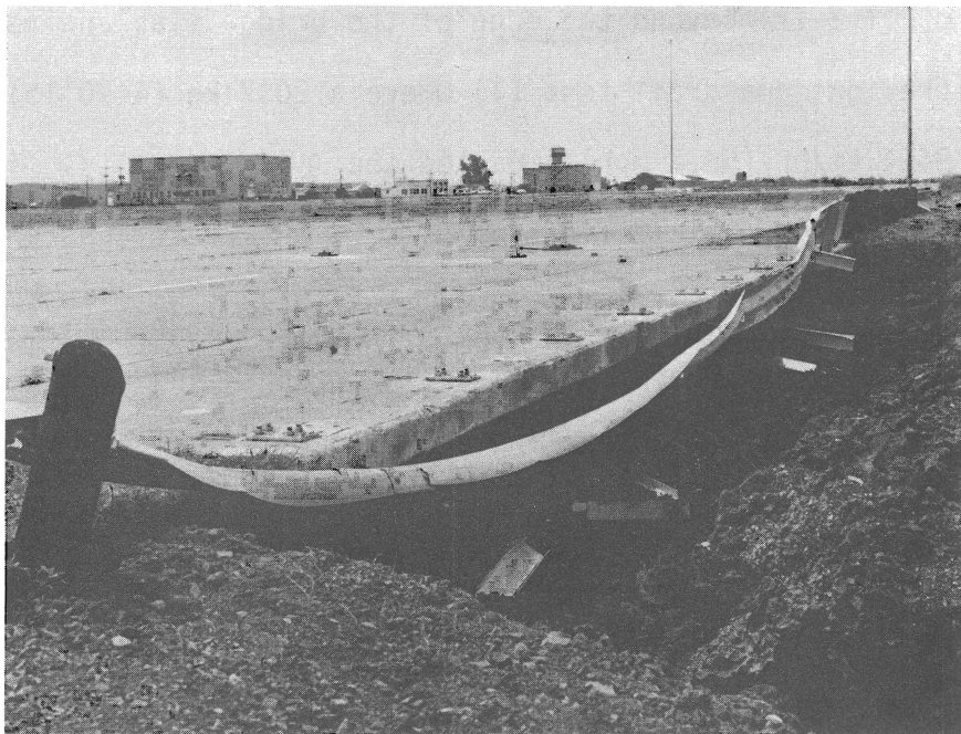
Figure 11. Closeup of Bridge Rail Damage after Test 1A.
