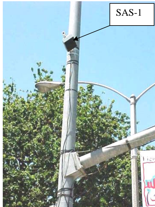
Figure 3. SAS-1 Mounting Location for Tests by City of LA.
