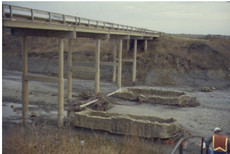
Figure 11.16. Exposed Piers on the North Sulfur River.
