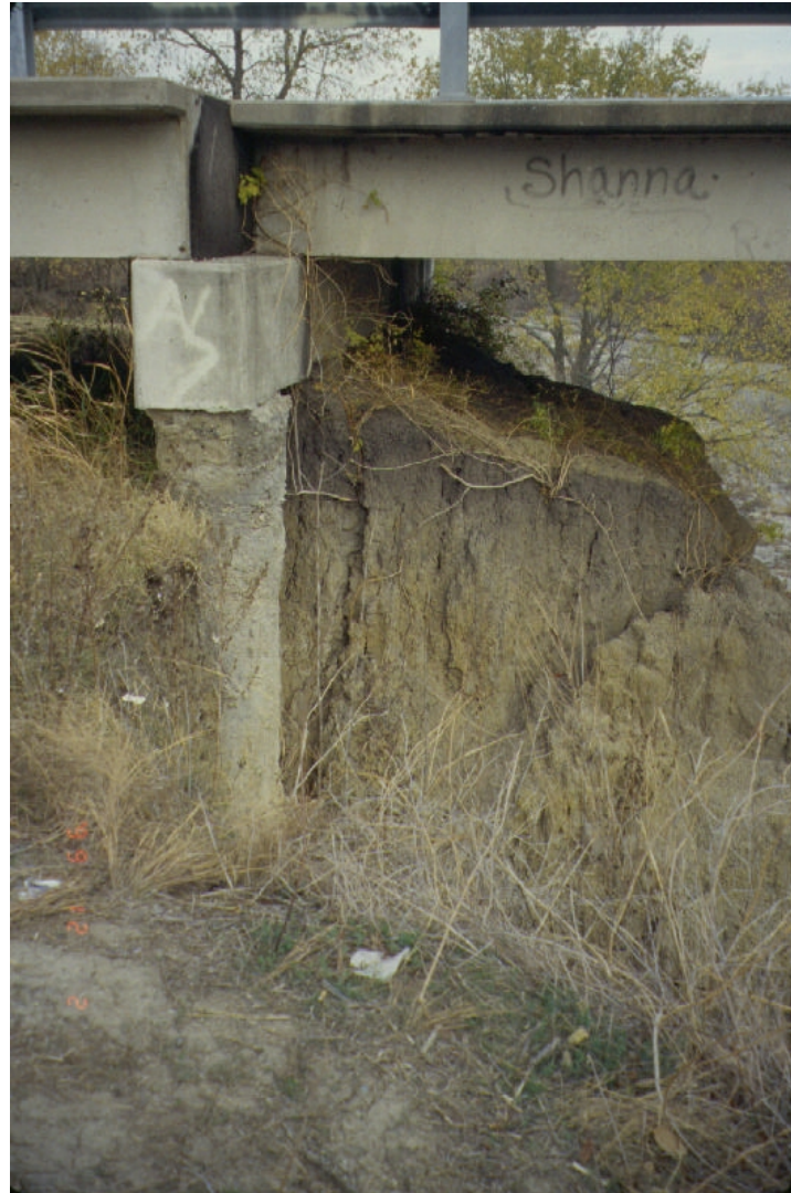
Figure 11.17. Erosion of Abutment on the North Sulfur River.
