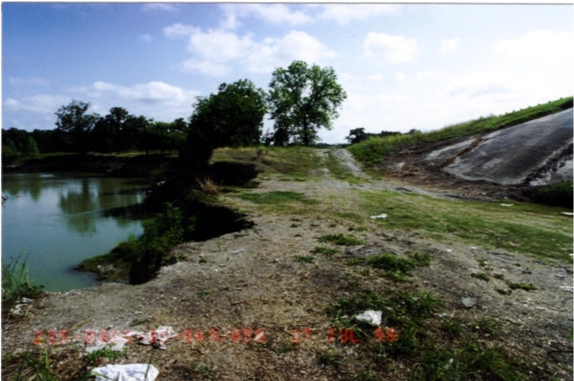
Figure 11.26. Bank Erosion near U.S. 59 at Guadalupe River Bridge.
