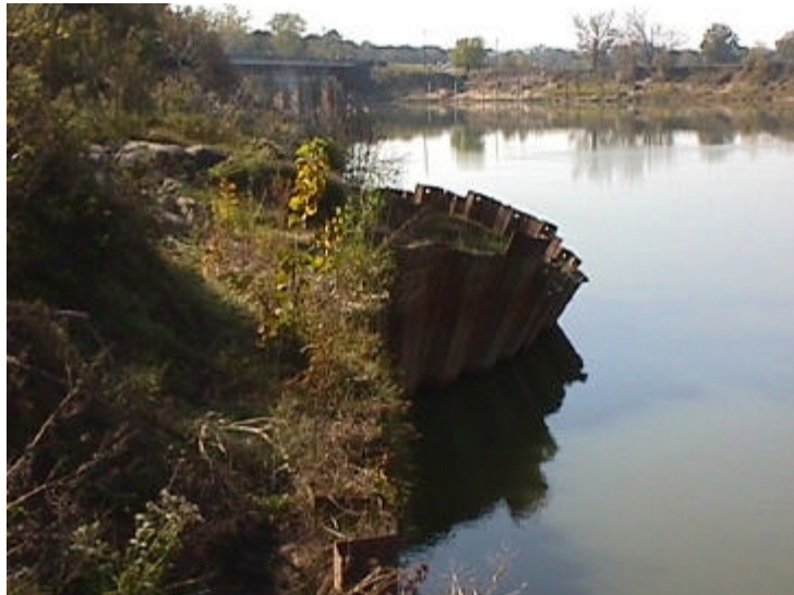
Figure 11.13. Failure of the Sheet Pole Wall as a Countermeasure.
