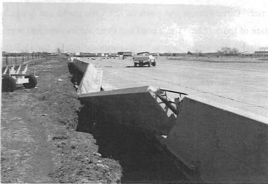
Figure 42. Post test damage to installation 1959A-5.
