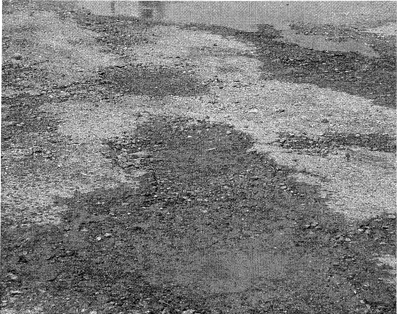
FIGURE 12. Additional Asphalt-Damaged Surface
