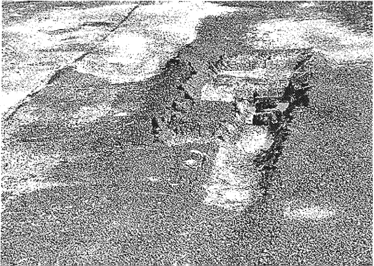
FIGURE 11. Example of an Apron Pavement Failure
