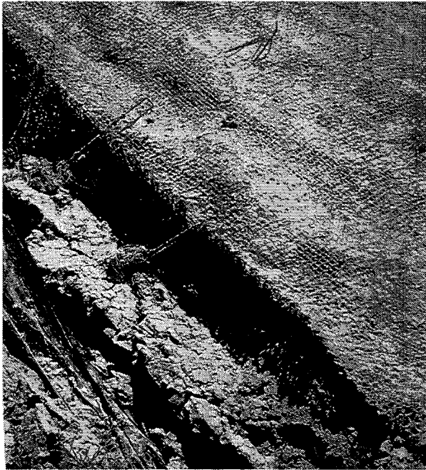
Figure 25. Washout at the Edge of the Belton Dekowe® 700 Plot
