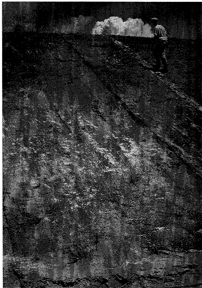
Figure 26. Damaged Belton Dekowe® 700 Plot
