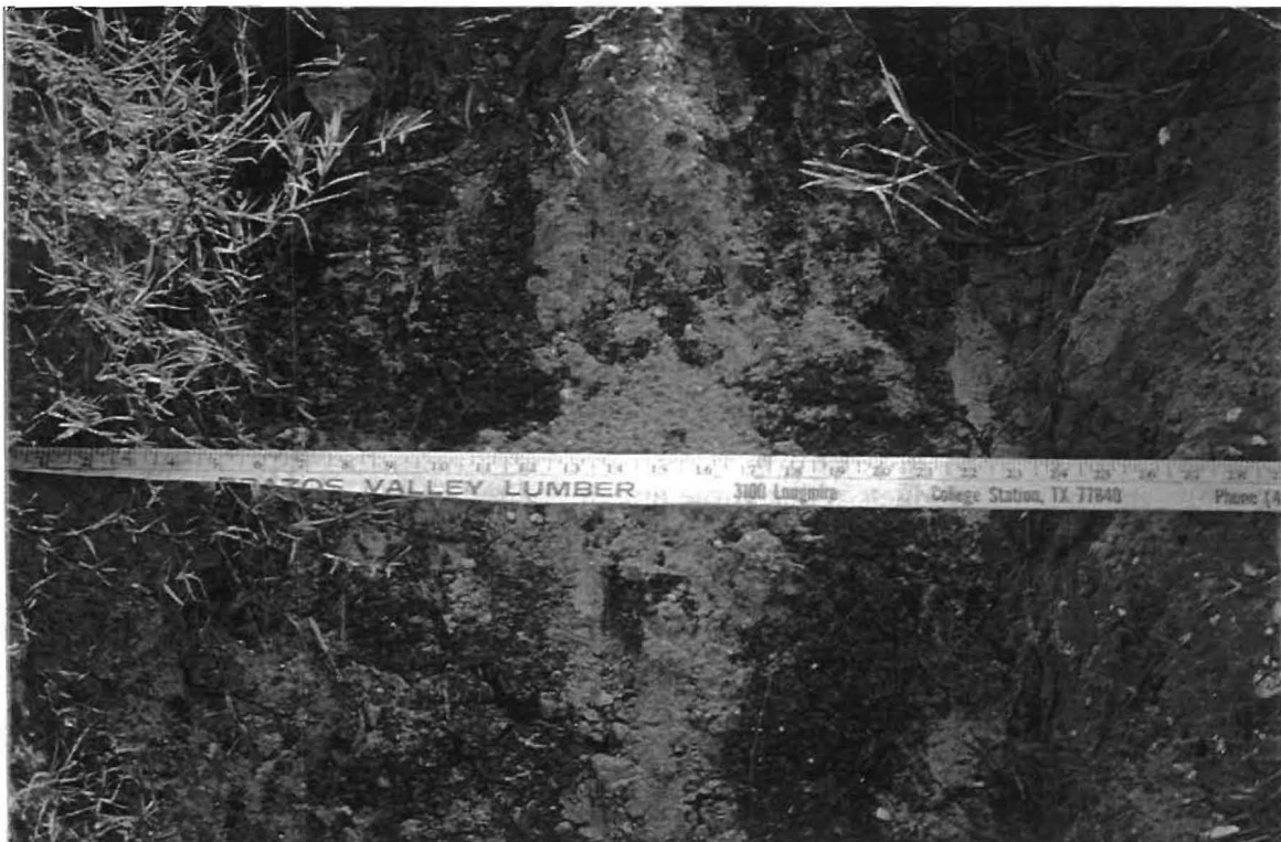
Figure 50. Washout of the 6' cap on the 2:1 Sand CONTROL plot
