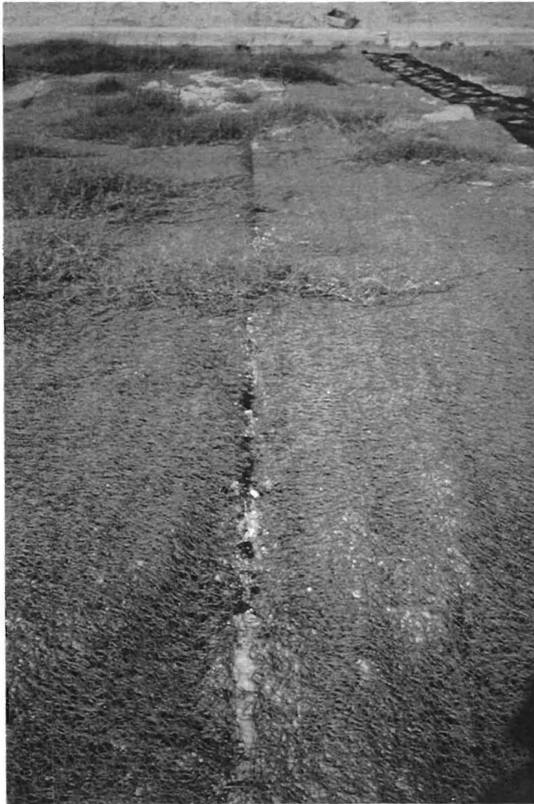
Figure 51. Seam separation on a 2:1 Sand PVC product plot
