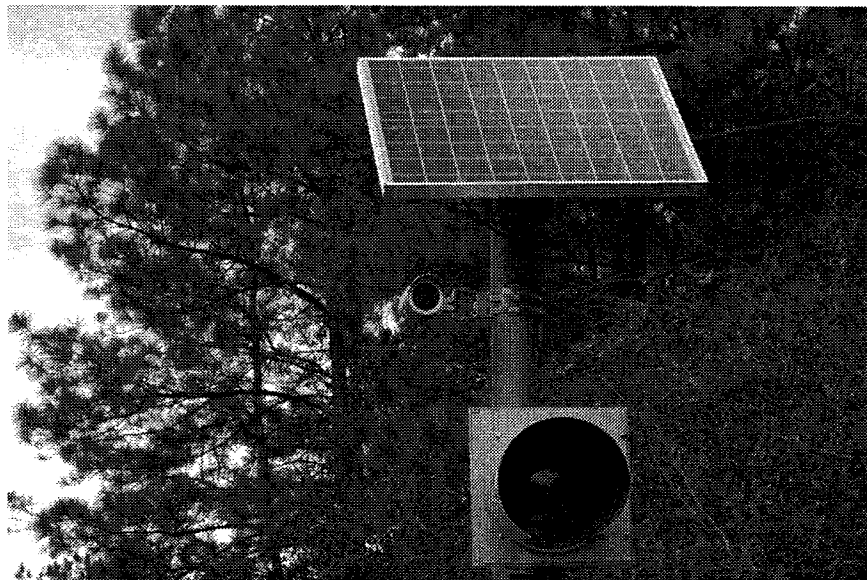
Figure 2-7. Solar Panel, Detector, Flashing Beacon Enhanced Sign Equipment.
