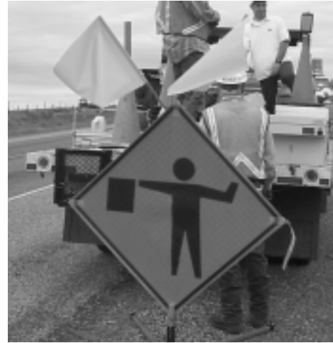
Figure 38. Fluorescent Orange Signs.
