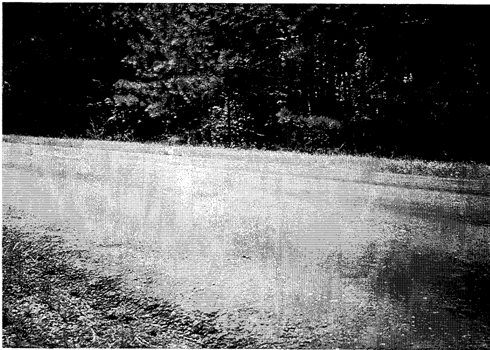
Figure 23. Kilgore Test Section 1: Treated RAP (Rutting Distress).
