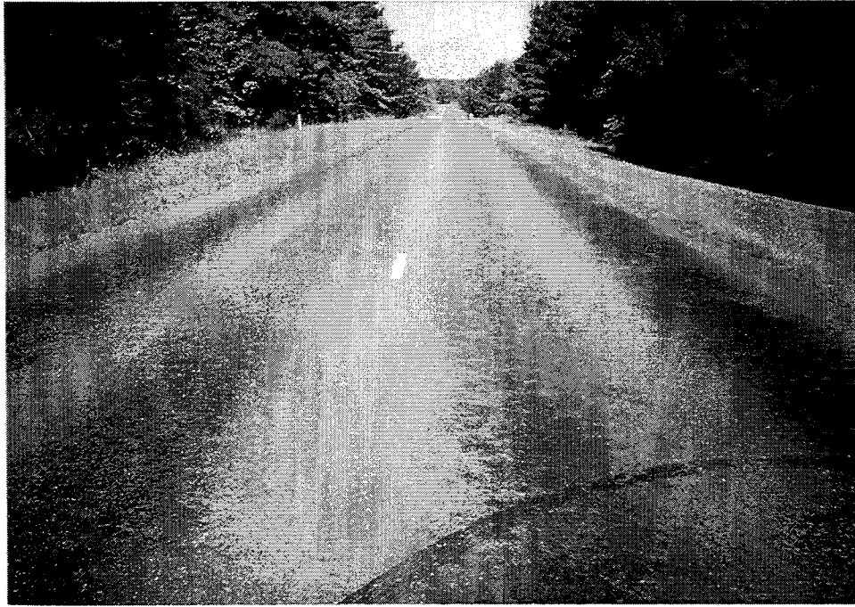
Figure 22. Kilgore Test Section 1: Treated RAP (Flushing Distress).
