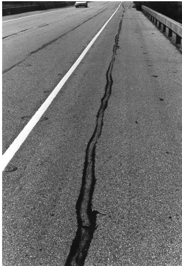
Figure 8. Asphalt Surface Cracking – Oso Creek/SH 286 Bridge (Overall View).
