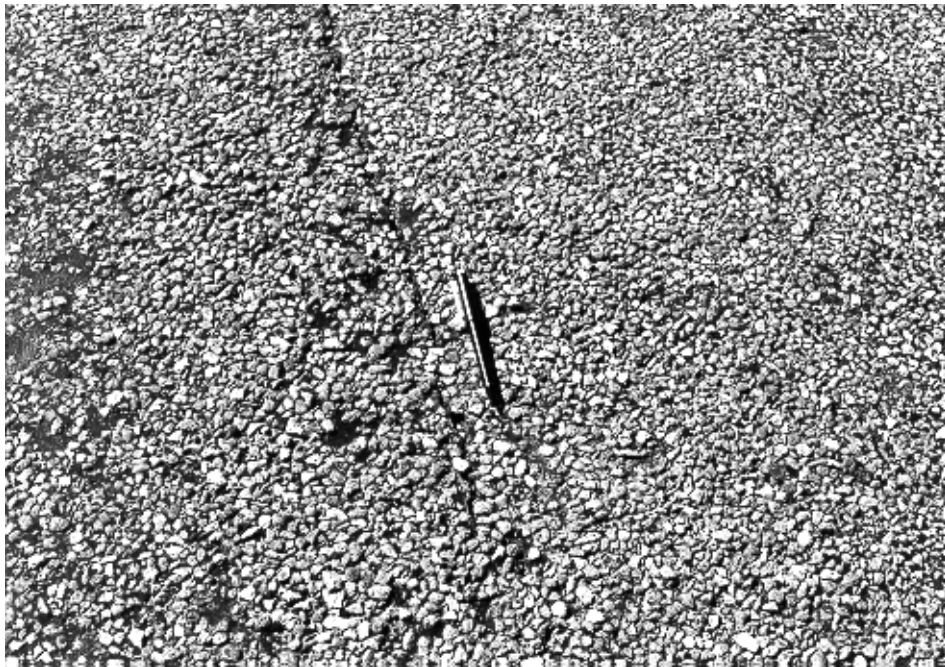
Figure 6. Asphalt Surface Cracking – Quinta Creek Bridge.
