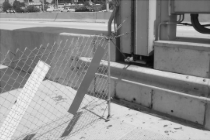
Figure 3-18. Wire Mesh Restraining Barrier.
