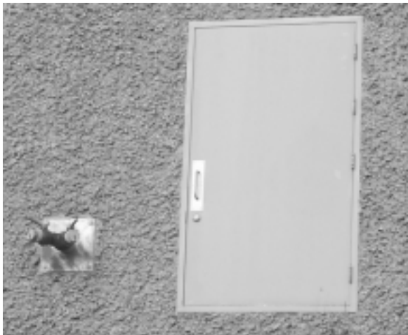
Figure 9-3. Fire Hydrant in Sound Reduction Wall.
