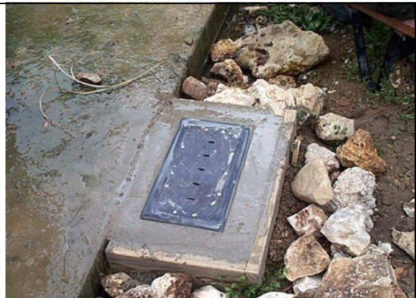
Non-boxed Effluent Sampler.
