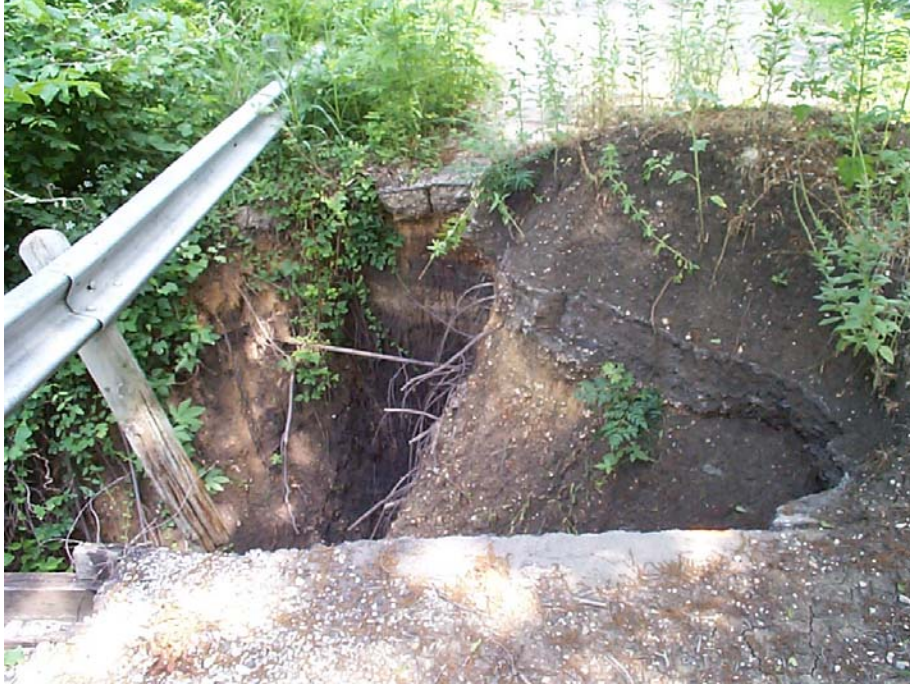
Figure 4. Erosion Caused by Flow in Drainage Swale.
