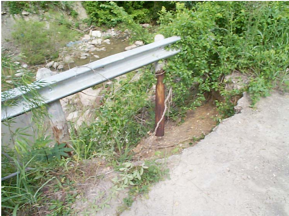
Figure 2. Failure on Roadway Embankment.
