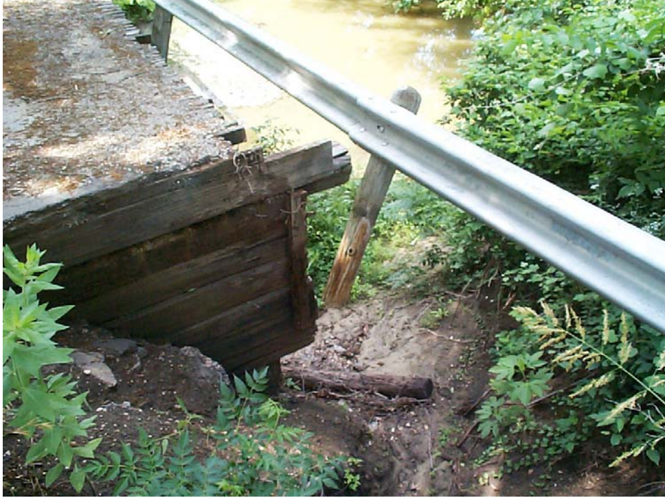
Figure 1. Failure Near Abutment Area.
