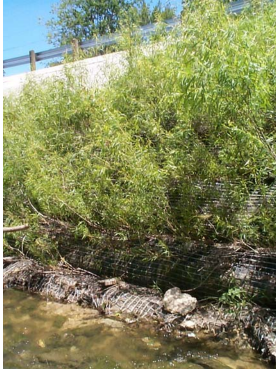
Figure 14. Low Survival on Bottom Layer of Cuttings.
