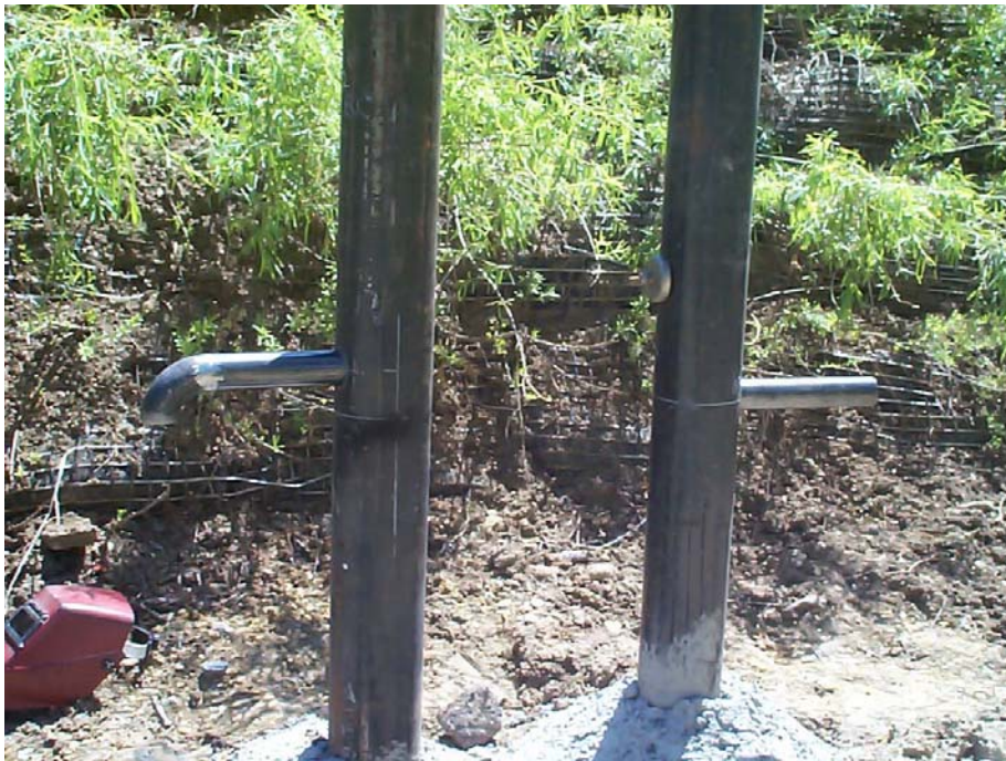
Figure 13. Monitoring Standpipes: Right Records Pressure and Velocity Head; Left Records Surface Water Elevation.
