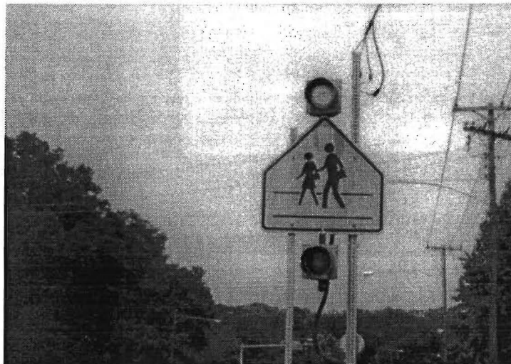
Figure 5-42. School Crossing Sign with Wig Wags in Tyler, TX.
