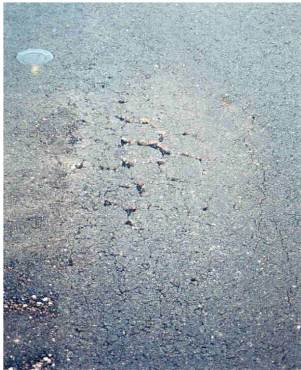
Figure 16. Alligator Cracking 2 Days after Construction.
