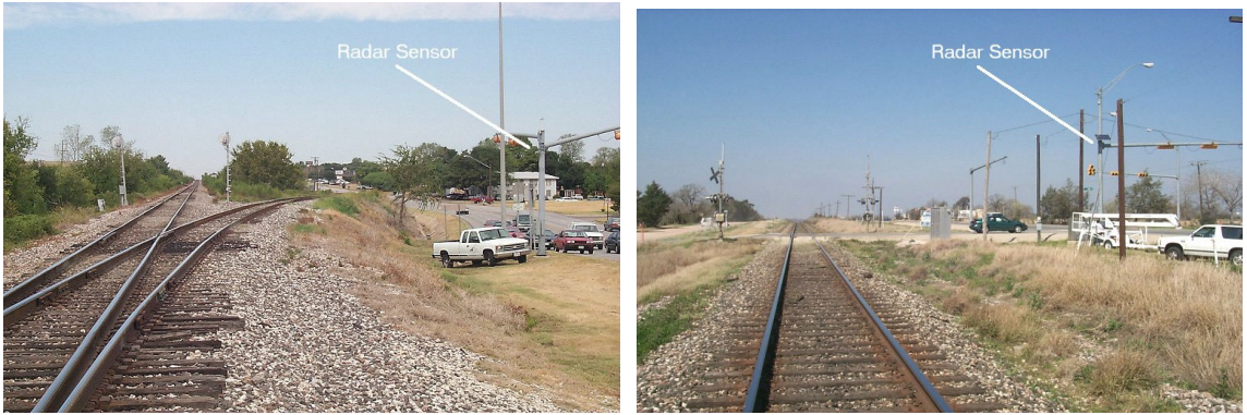
Figure 3. Sample Sensor Installations.
