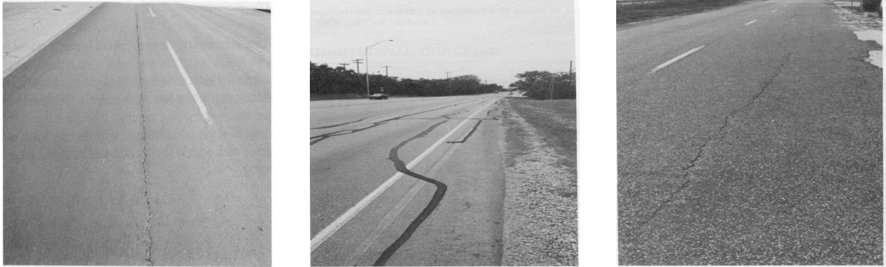
Figure 3. Examples of Longitudinal Cracking (TxDOT, 1998).
