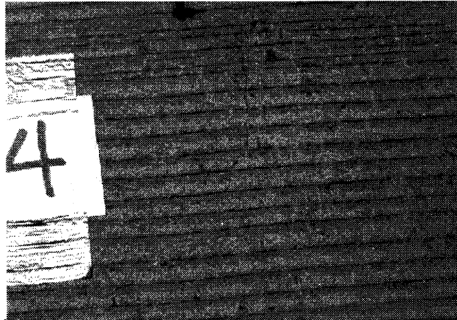
Figure 2.7. Longitudinal Deck Cracking on US 180 Bridge.
