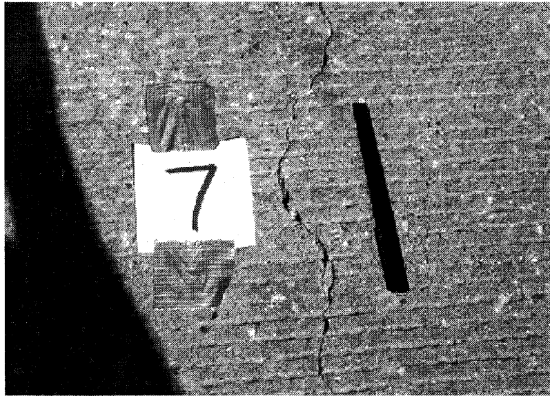
Figure 2.10. Longitudinal Deck Cracking on FM 730 Overpass.
