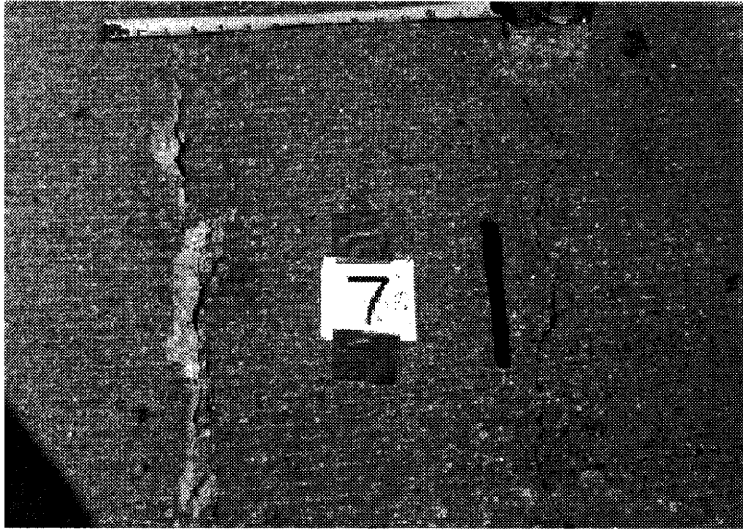
Figure 2.10. Longitudinal Deck Cracking on FM 730 Overpass (continued).
