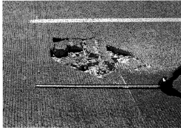
Figure 2.5. Deck Blowout on FM 660 Overpass.
