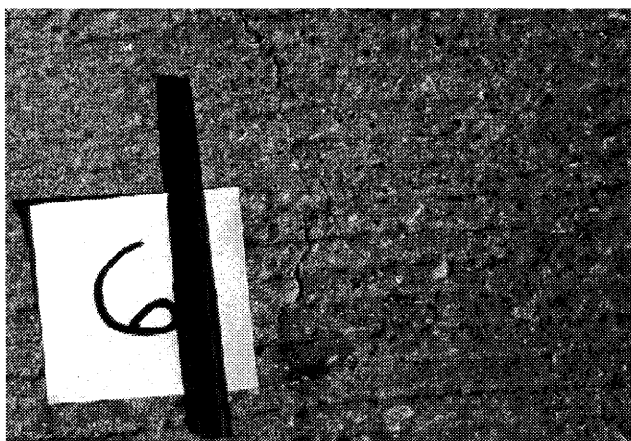
Figure 2.9. Longitudinal Deck Cracking on FM 51 Overpass.
