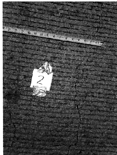
Figure 2.4. Longitudinal Deck Cracking on FM 660 Overpass.
