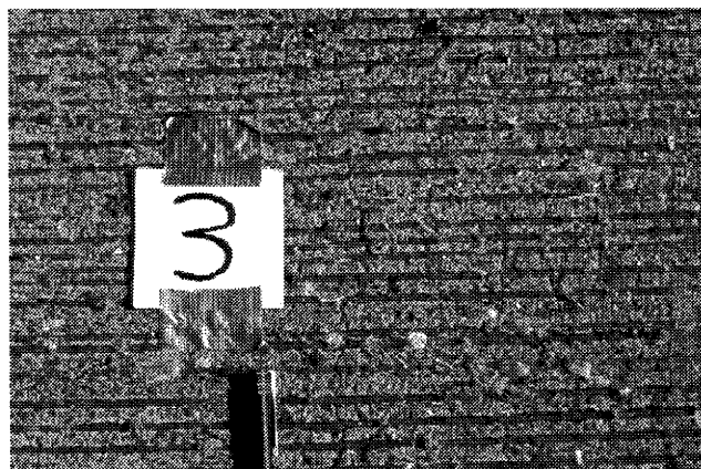
Figure 2.6. Longitudinal Deck Cracking on Cooper Street Underpass.
