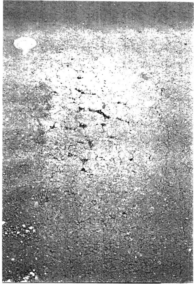
(b) Failed Section Which Occurred Either Side of Longitudinal Joint.
