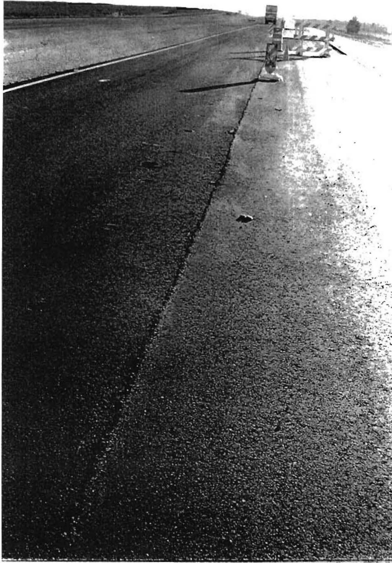
(a) Suspect Longitudinal Joint.
