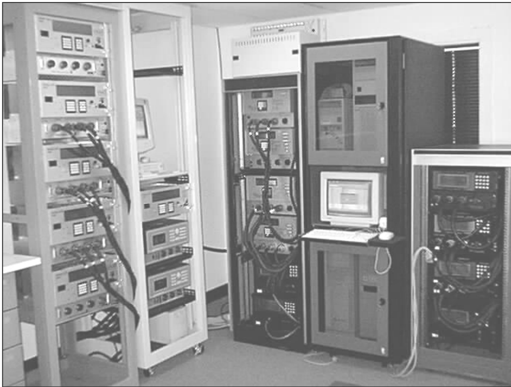
Figure 7. TransLink ® Roadside Equipment Laboratory.
