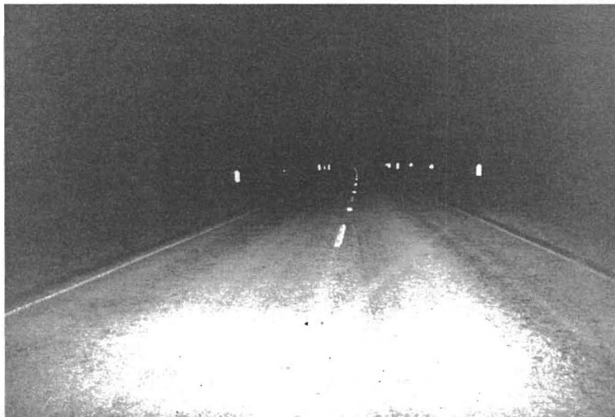
FIGURE 2-6. Type OM-2 Object Markers, Post-Mounted Delineators, and a 65-Meter Segment of Edgeline Approaching the Bridge Ends
