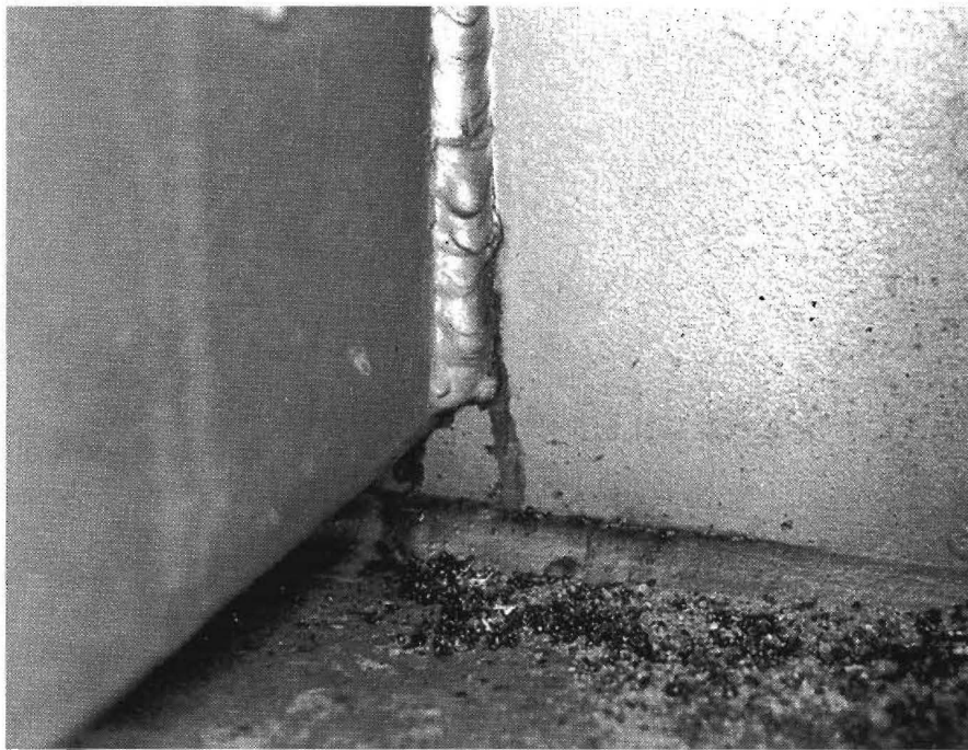
Figure 1-2: Fatigue crack at end of unstiffened web gap of diaphragm connection plate.
