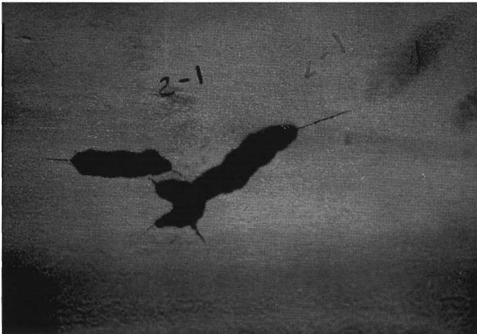
Figure 3-10: Examination of crack using dye penetrant.
