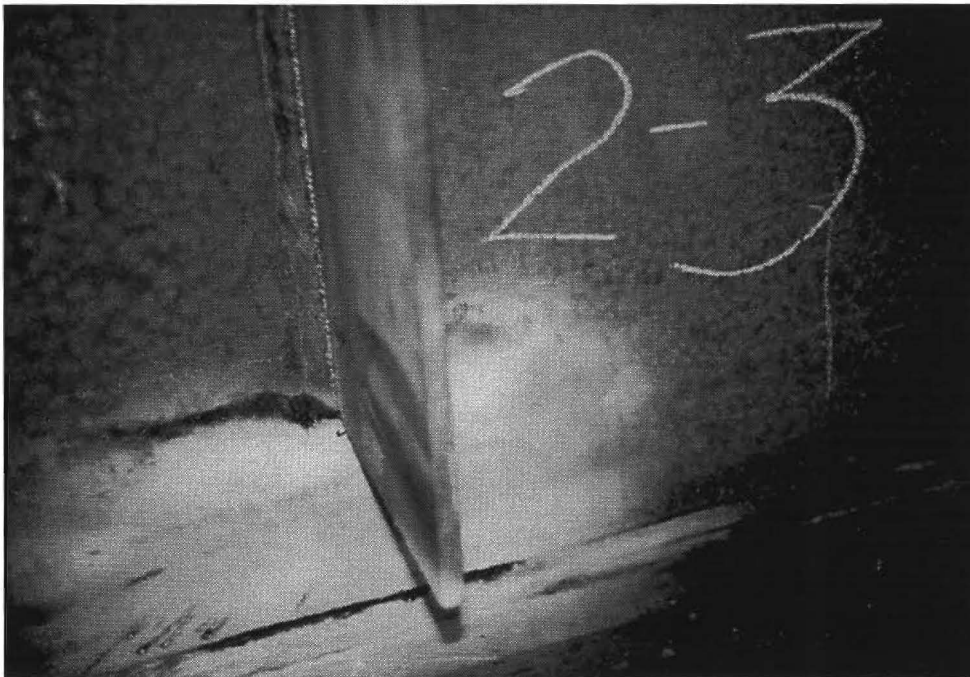
Figure 3-20: Examination of crack using dye penetrant.
