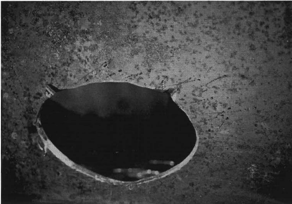
Figure 3-27: Flame-cut hole in web plate at Stiffener 1-2.
