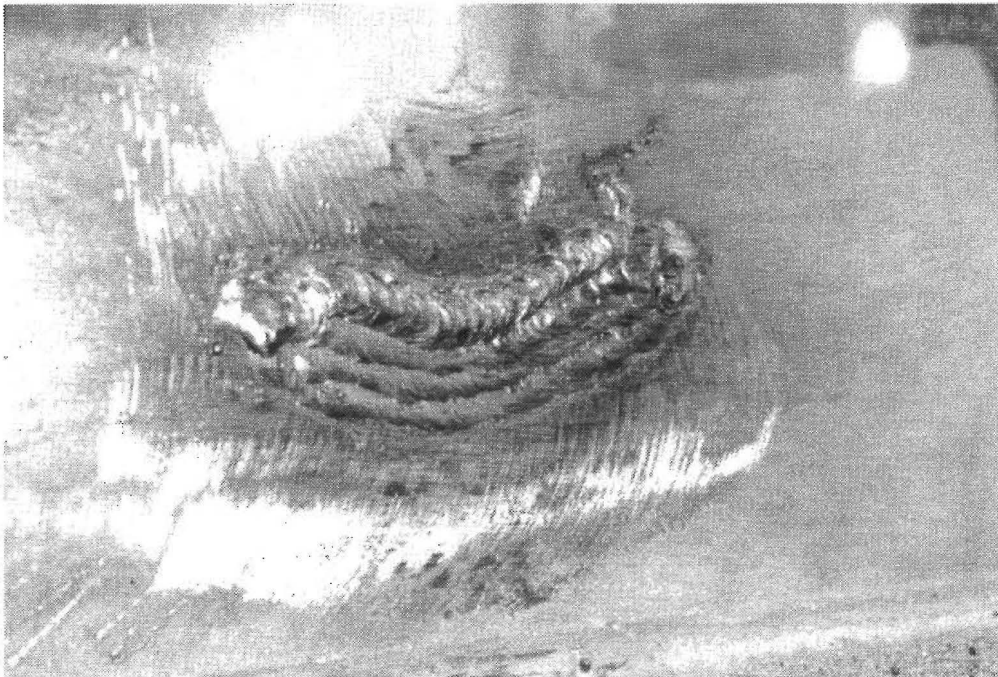
Figure 3-31: View of re-welded fatigue crack lines.
