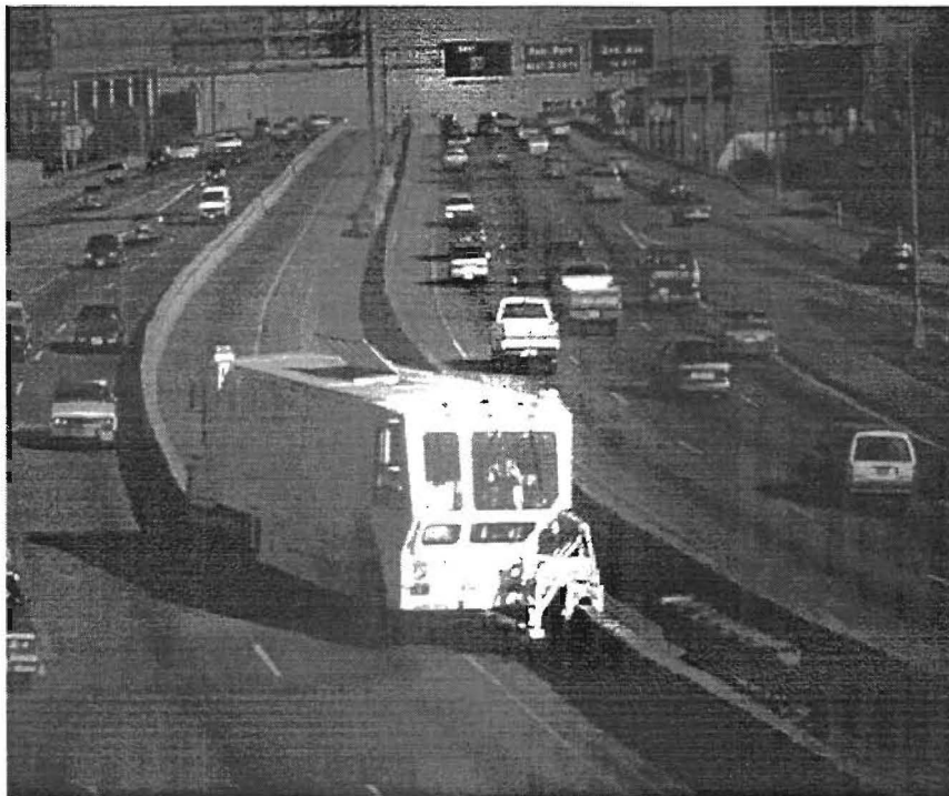
Figure 7. Machine Used to Shift the Moveable Concrete Barrier on East R.L. Thornton
