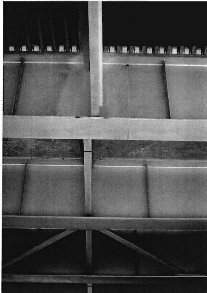
Figure 2-9: View of Girder No. 5 connection plate offset, Westbound Structures.
