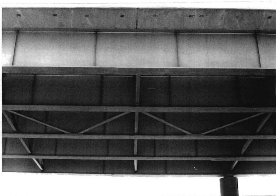
Figure 2-8: View of Girder No. 5 offset, Westbound Structures.
