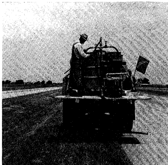
Figure 5. Post-surface applications were made using a sprayer developed by the Texas Highway Department. This spray unit utilizes a water tank as a herbicide container and incorporates a system which includes a pump, a pressure regulator, a bypass, and a boom with nozzles for distribution of the spray solution.
