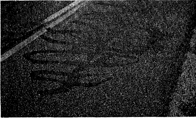
Figure 16. Flexure and deformation cracks on State Highway 283 north of Crowell.
