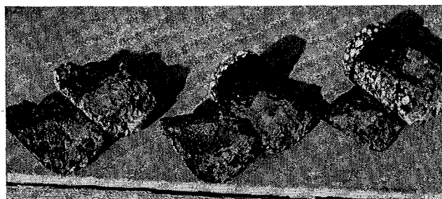
(b) Cores taken from treated and untreated portion of the reflected crack.
