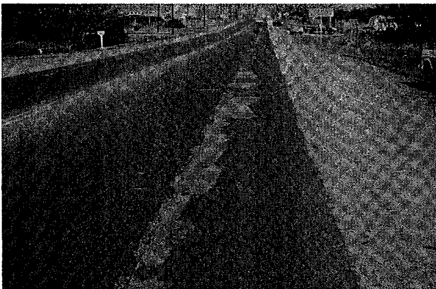
Figure 13. Cracking problem for which fiber mat was used (U. S. 190 east of Bryan, Texas).
