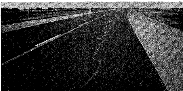
Figure 18. Longitudinal cracks caused by dry weather shrinkage.
