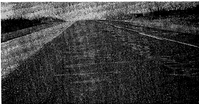
Figure 17. Flexure and deformation cracking in the wheel paths on State Highway 283 north of Crowell.
