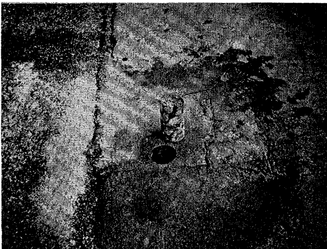
Figure 1. Concrete area of distress adjacent to a construction joint in CRCP (core upside down to view honeycombing).
