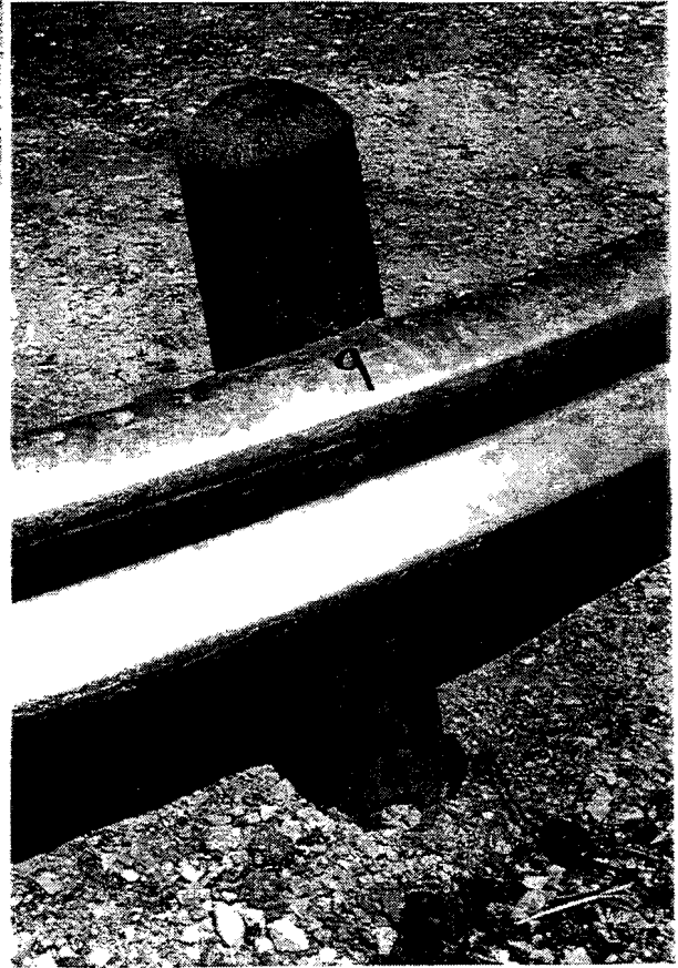
FIGURE F-95. Damage at posts 8 and 9, Test 1263-6
