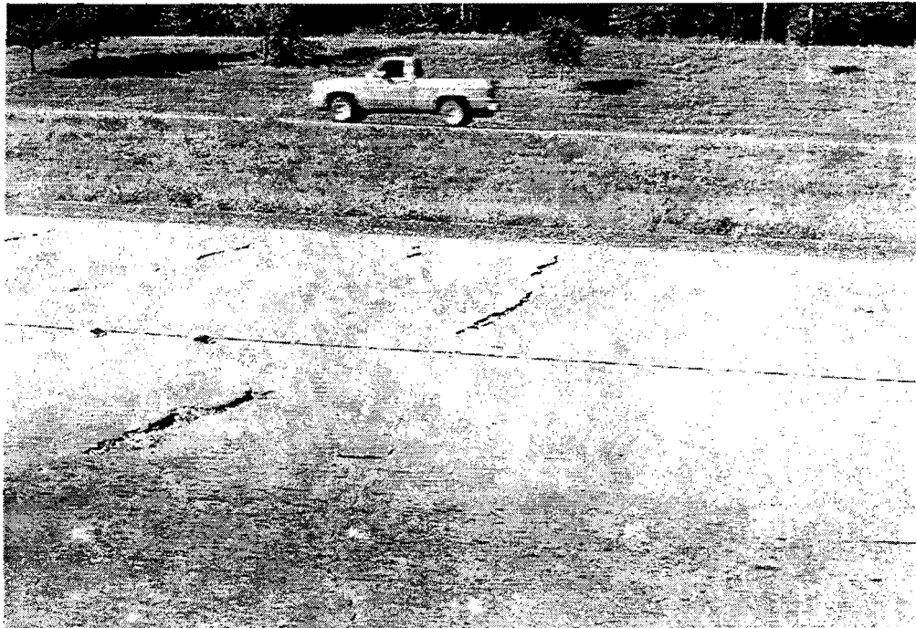
FIG. 1. Typical Spall in Concrete Pavements
