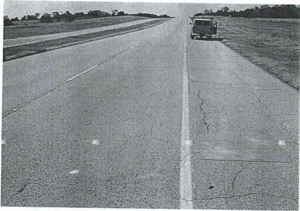
Figure 25. Photograph of US 82 west of Sherman, Texas, Part of the 10 Mile Section Being Evaluated for Pavement rehabilitation. This Section is the Original Surfacing, Now 20 Years Old.
