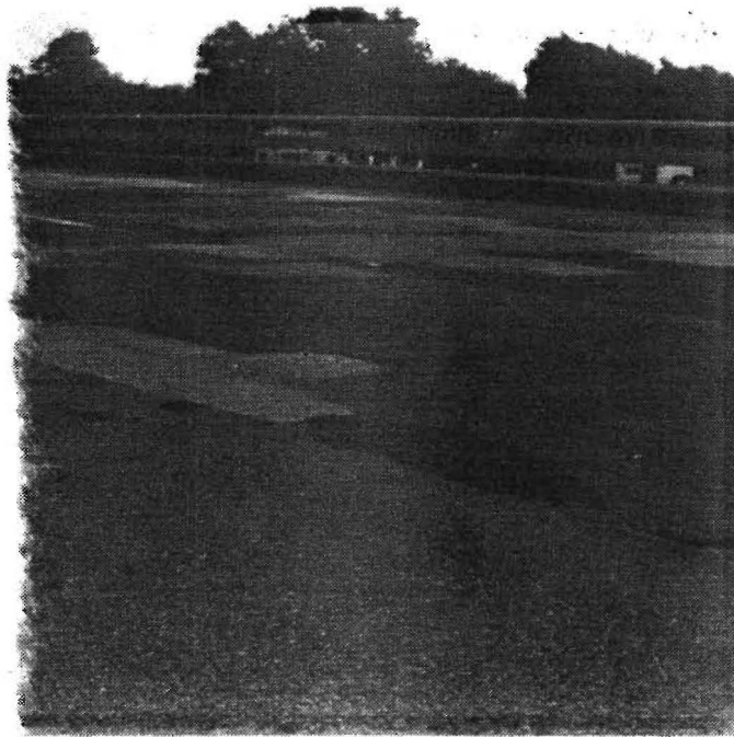
Photo # 1 -- Inadequacy of Sufficiency Rating as a Measure of Deficiency
