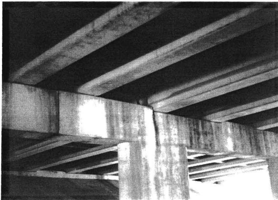
Photo # 11 -- Underside of Bridge Deck (Falling Seals)
