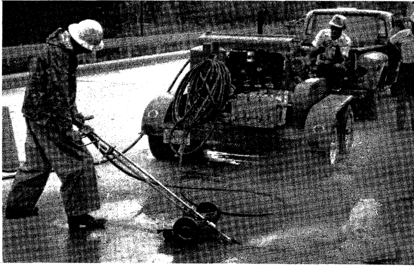
Fig. 15. After conducting limited experimental joint cleaning in this study the Beaumont district accomplished a major joint cleaning program.
