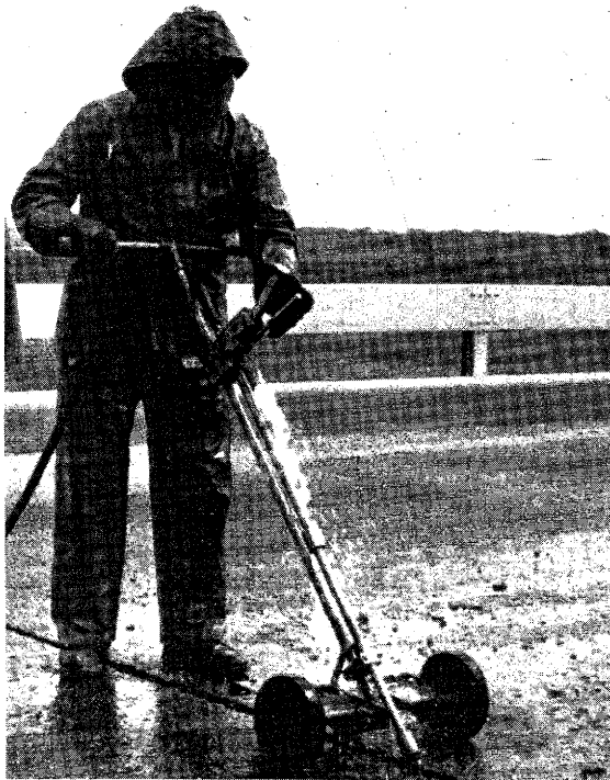
Fig. 9. To make operations easier a small cart was built that opposed the thrust of the jet stream.
