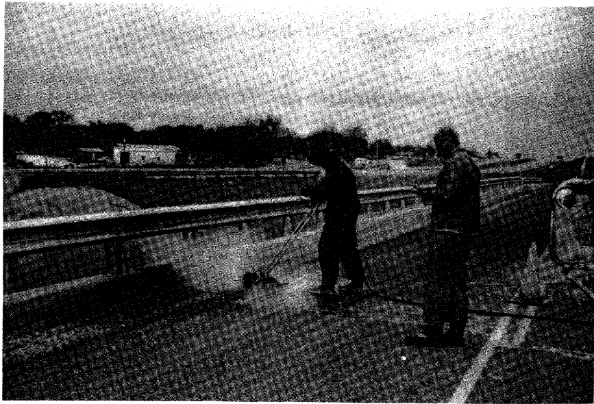
Figure 5: High-pressure water-jet being used to clean debris from joint. The jet "gun" has been mounted on a cart to facilitate operations.
