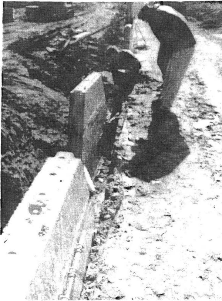
Figure 7.1 Initial separation of facing units
