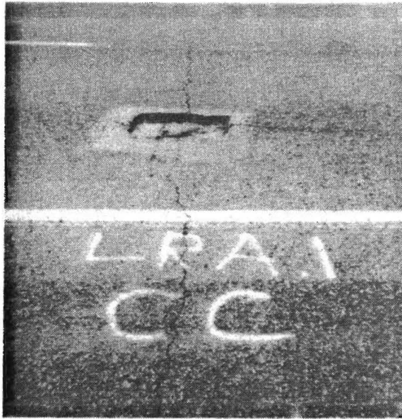
Pothole "prepared" with tack coat
