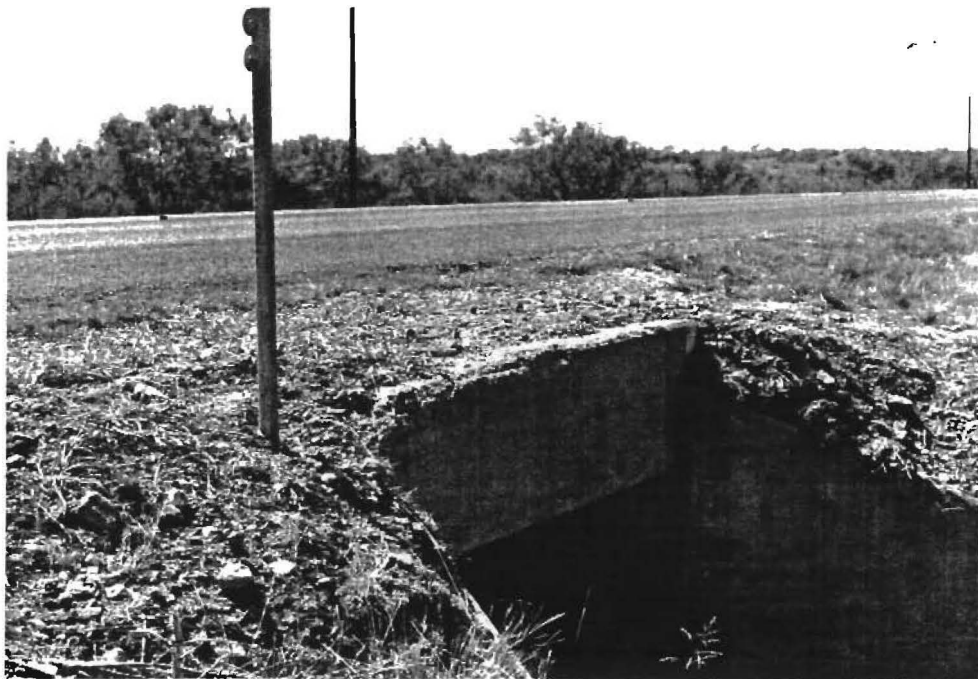
Figure 3: Headwall Broken Off at Ground Level
