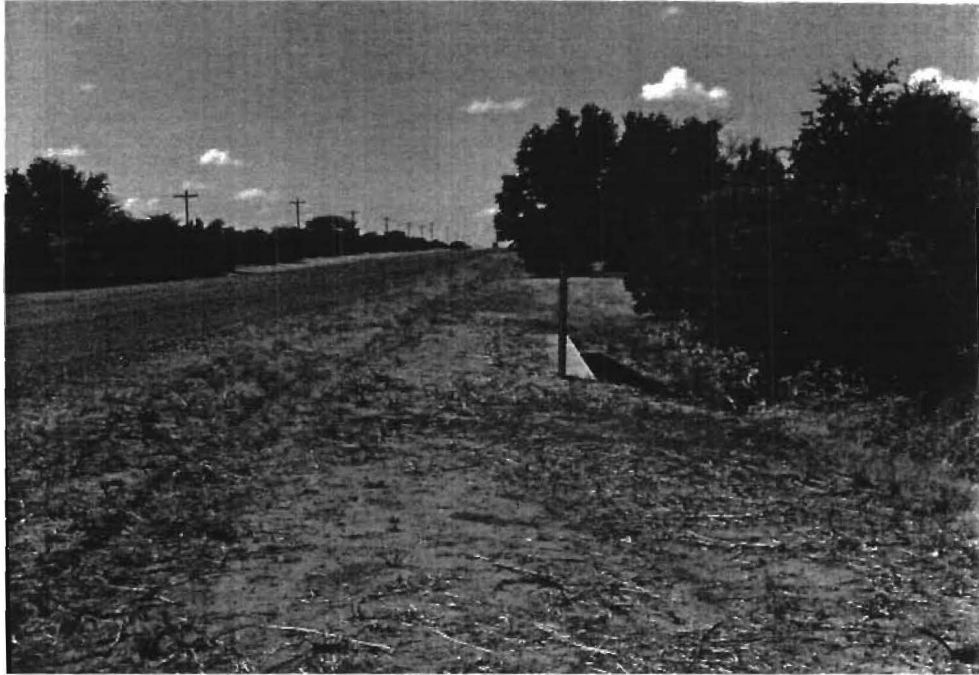
Figure 4: Headwall with Fill Added to Bring Ground Level up to Top of Headwall
