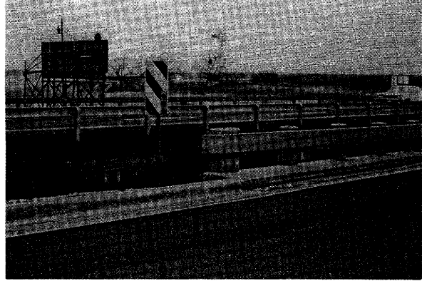
b. Open Gap Between Parallel Bridges (Code 12-01)
