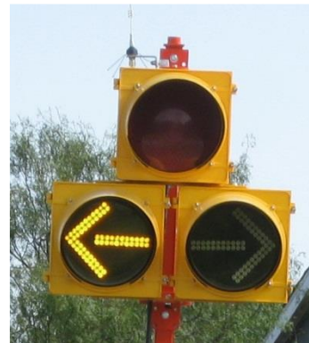
b. Flashing Proceed Indication.
